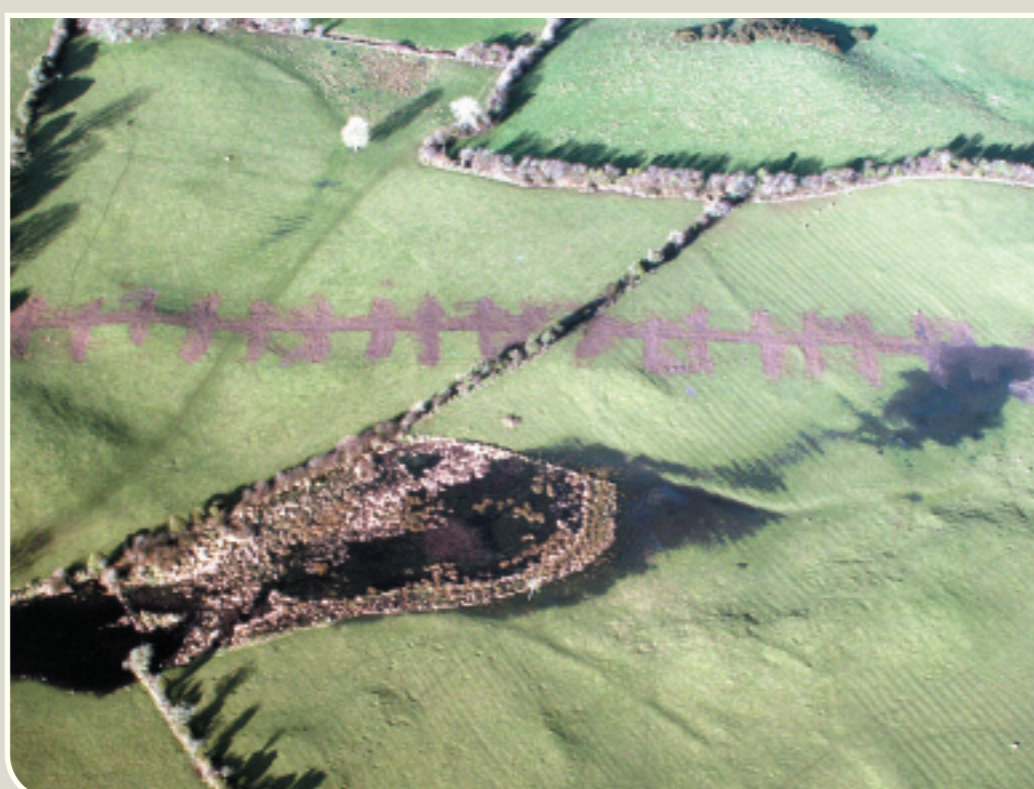
Aerial view of centreline test trenching carried out on the scheme. (Photo Markus Casey)
